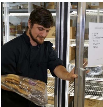
Refrigerators/freezers to store perishable rescued surplus food
